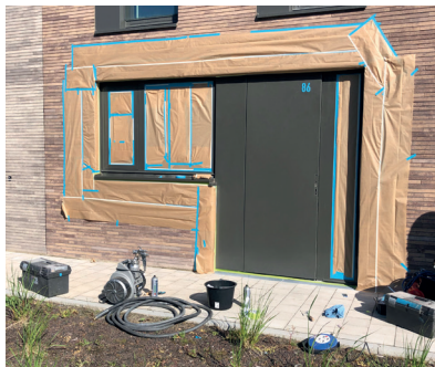
Figure 3.32: Protecting parts that are not being painted at the same time. © Respirepair
